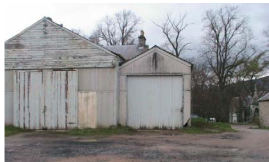
Fig. 3 : former bus garage – roof and chimney of bus station house visible above roofline.
